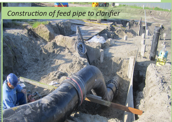
New discharge infrastructure for effluent, sludge recycling and floating sludge evacuation
